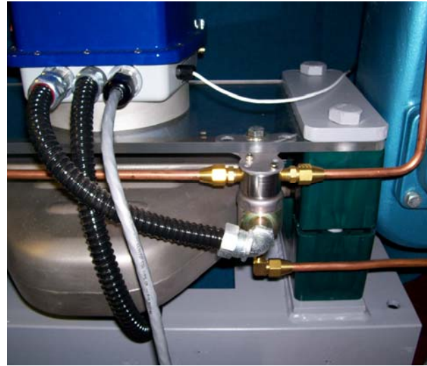
Figure 4-8. Valve Wiring and Plumbing
