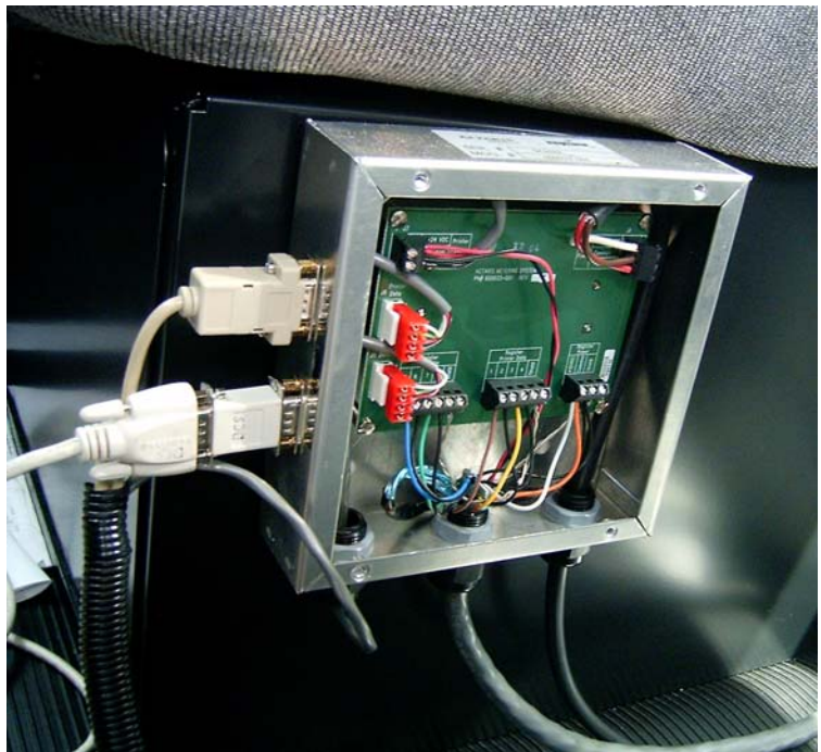
Figure 4-12. Junction Box Installation
