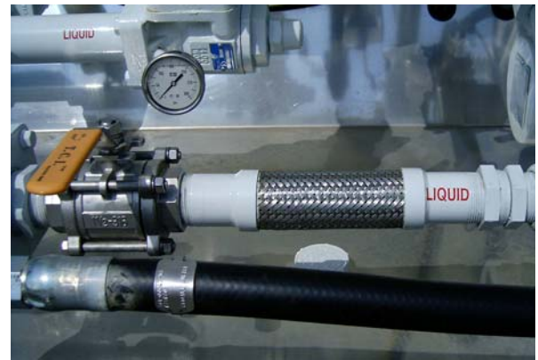
Figure 4-3. Flexible Hose at Outlet
